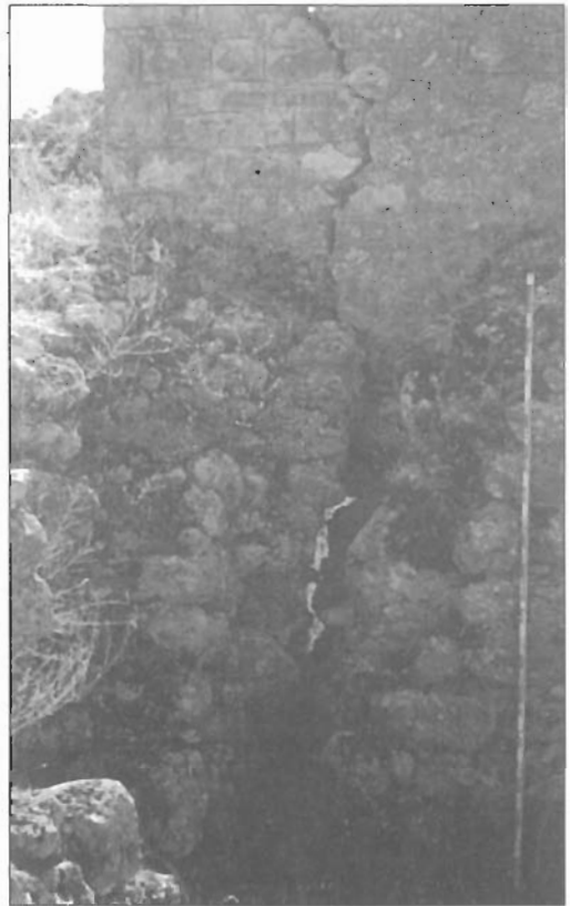
Fig. 5: Active fracture within the the superstructure. 2-3 m. scale bar. For location see fig. 2.
