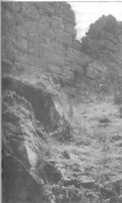
Fig. 4: Fault within the Mendenitsa horst, affecting the superstructure. For location see fig. 2.
