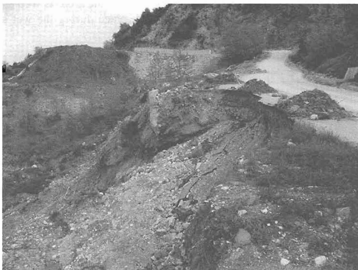
Figure 3 - Landslide No1 (cross-section AA')
