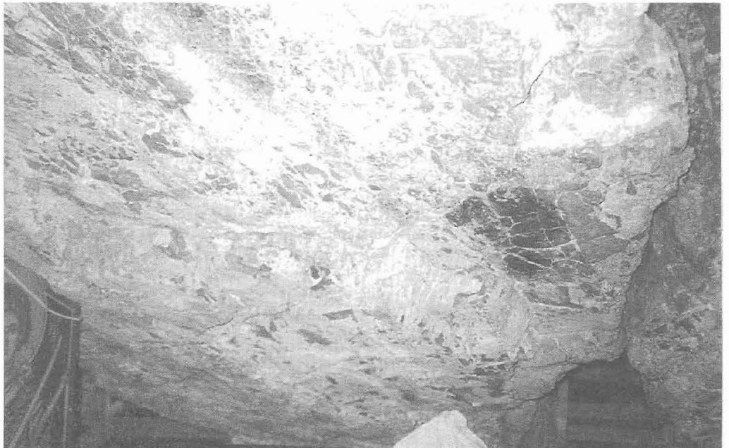
Figure 8 - View of the wedge formed by the faults intersecting the cave. The concrete column constructed for the support of the wedge is visible on the left side of the figure
