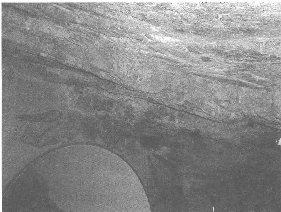
Figure 6 - Ceiling view of section A. Unsupported Section. This picture clearly presents a side view of the arc supporting section D, covered by hagiography
