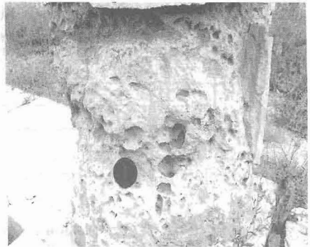
Figure 13 - Severe decay of bottom column piece constructed of type III sandstone and shape alteration
