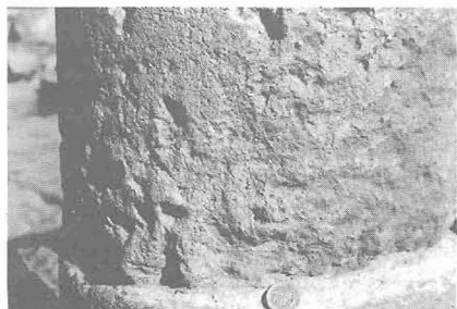
Figure 19 - decay form on sandstone type I
