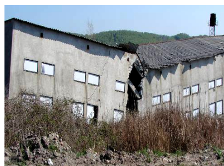
Photo 5: Building affected by the landslide, at Seciurile
