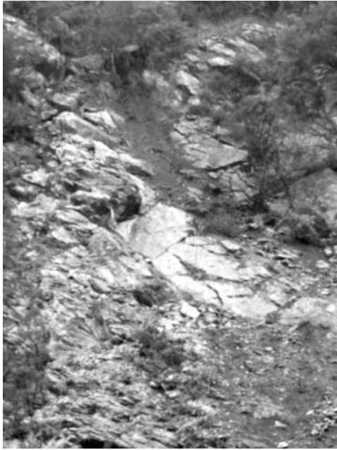
Fig. 6: The initiation of the slope failure originated as sliding along the joint 350/47.
