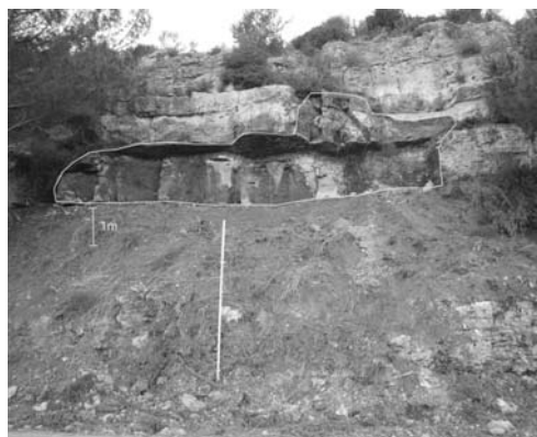
Fig. 3: Source area of the rock falls occurred on December 16, 2009.
