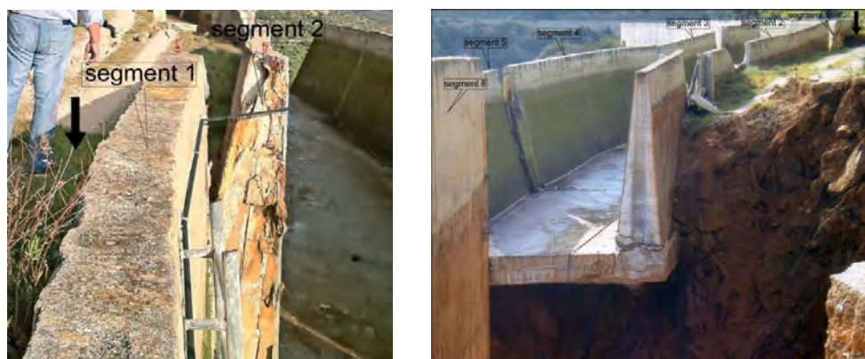
Figure 6 - Soil subsidence on the uphill side of the left canal wall between segments 1 and 2 and along the surveillance road.
