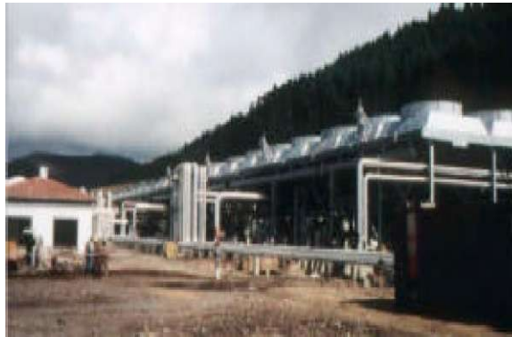
Ribeira Grande Binary Plant
