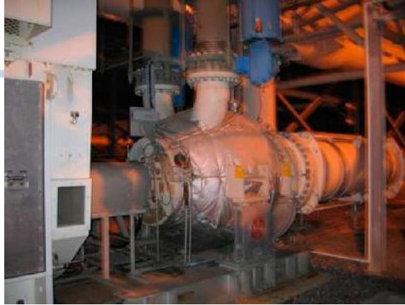
Salavatli Binary Plant
