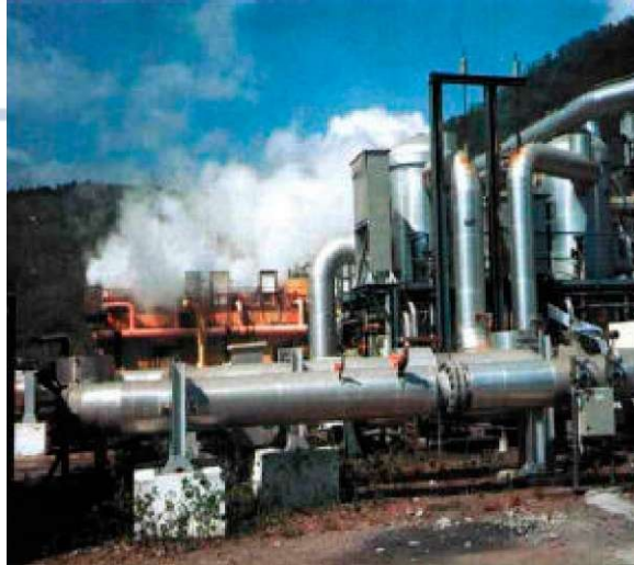
Bouillante Binary Plant.
