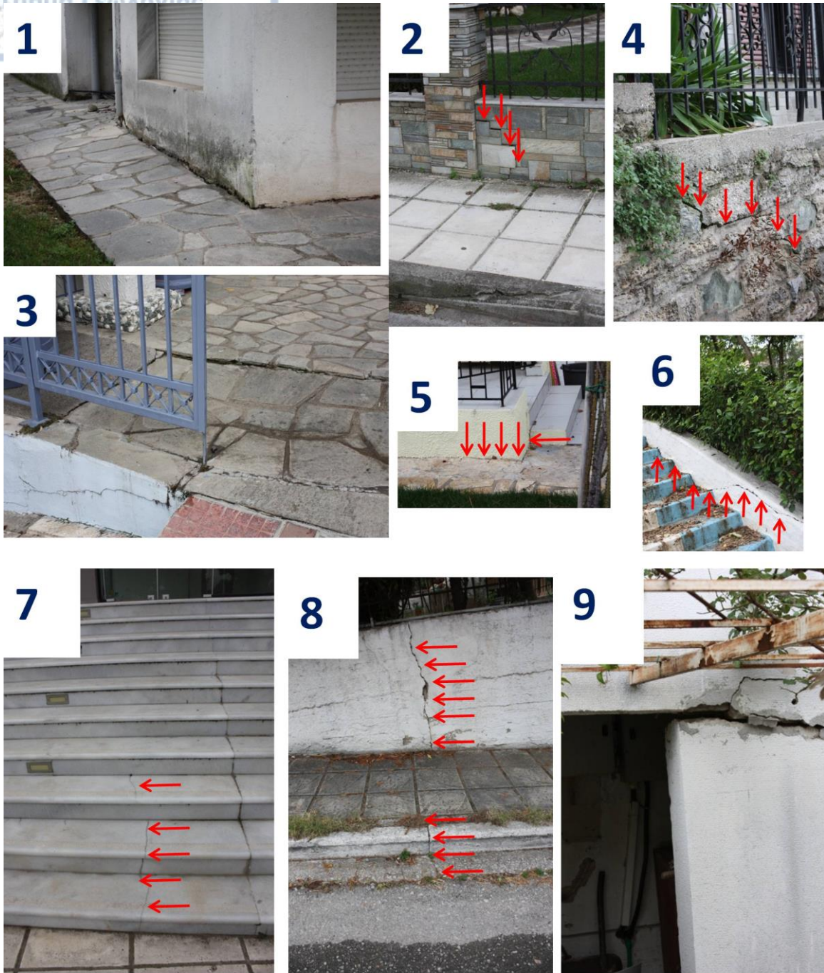
Figure 4.24 Failures detected at Perea at the areas where there are deformation point results during the ENVISAT monitoring. Red arrows in each image highlight the failures. Numbers of these images can be found also at the two inset maps of Figure 4.23.
