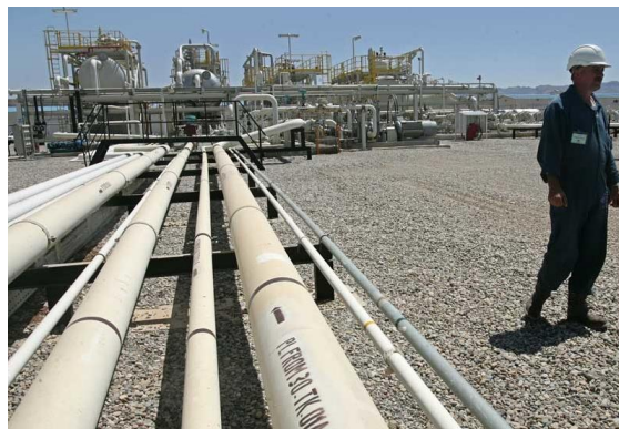
Figure 52: Receiving Facilities ( Source: www.oilandgasmiddleeast.com ).
