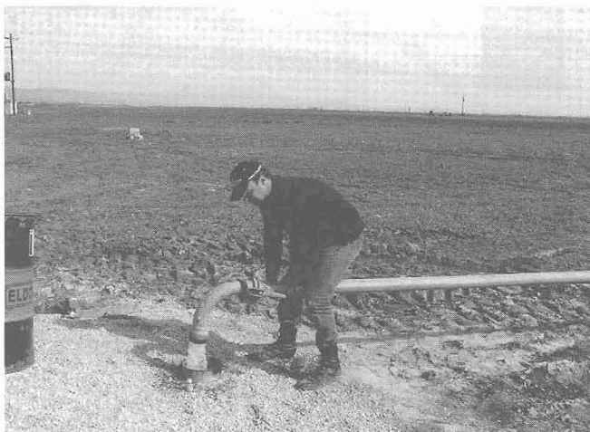
Figure 4 –Water recharge injection system
