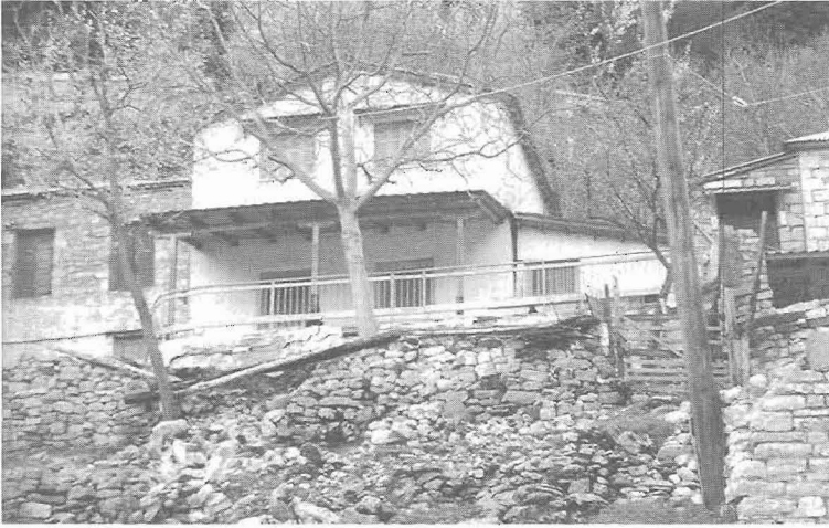
Figure 5 - A typical example of slope that failed during a year with prolonged high precipitation because of the increased loading of its crest. The landslide caused extended damages to the house
