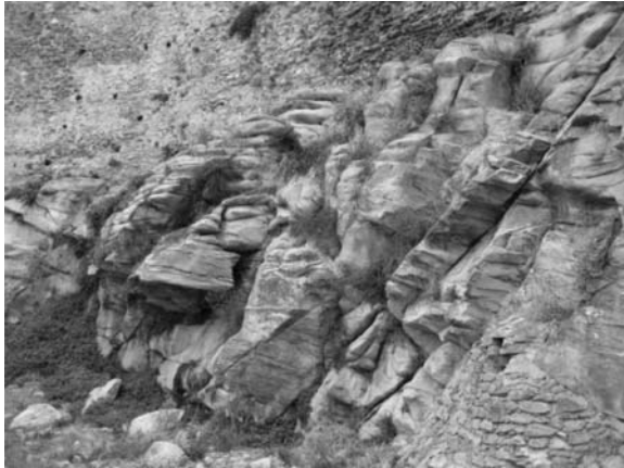
Fig. 6: Part P6. Several rock wedges are formed, to prevent them from sliding the underexcavated rock blocks were sub founded by the use of masonry walls – fills (lower right corner of the picture).
