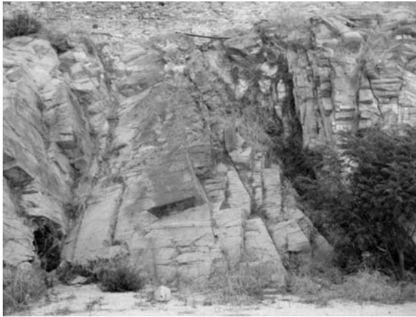
Fig. 4: Location P2. An oversized rock wedge that probably failed during the excavation of the small tunnel appearing at the base of the slope, on the left side of the picture. The extension of the failure could very easily damage the Byzantine wall.
