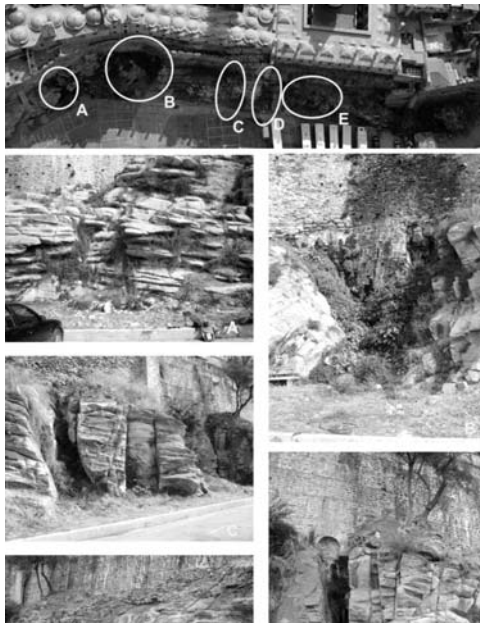
Fig. 5: Part P5. View of the slopes below Imaret monument intersected by the faults presented in the map of Fig. 1. The deterioration of the rock mass along the major tectonic lines cause serious rock slope stability problems threatening the monument. The letters pointing the various unstable locations correspond to the homonymous pictures (5A to 5E).
