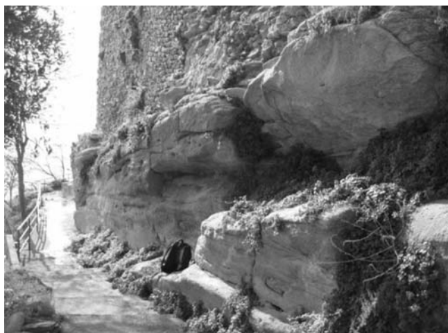
Fig. 8: Part P13. Underexcavated slope along a fault scarp. The wall was founded close to the edge. The toppling or the rupturing of the rock mass could cause extensive damages to the monument.
