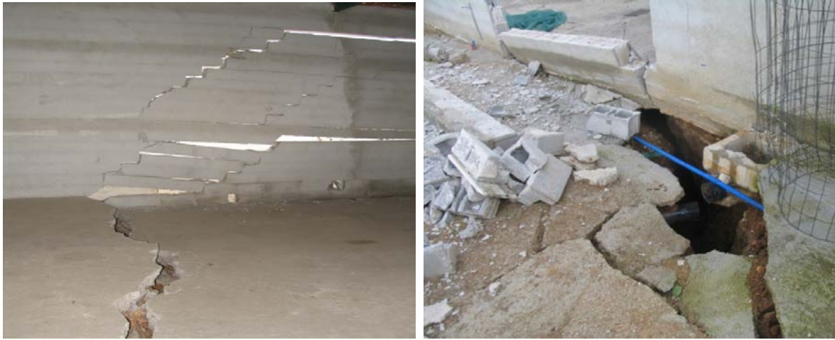
Figure 5.9 : Damages in house walls and house basis in Mavropigi residences.
