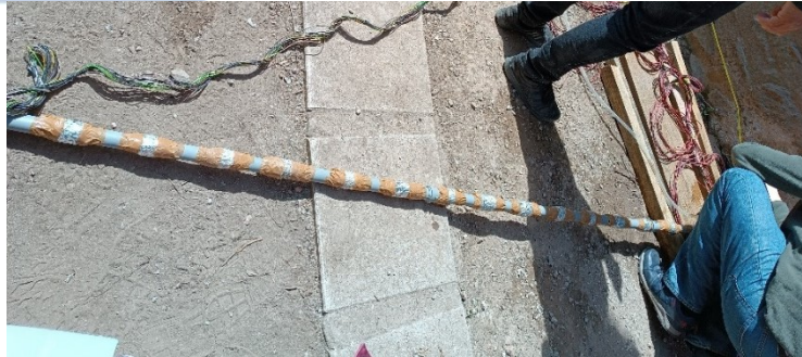
Figure 5.2: The PVC pipe construction that was used for the support of the borehole electrodes.
