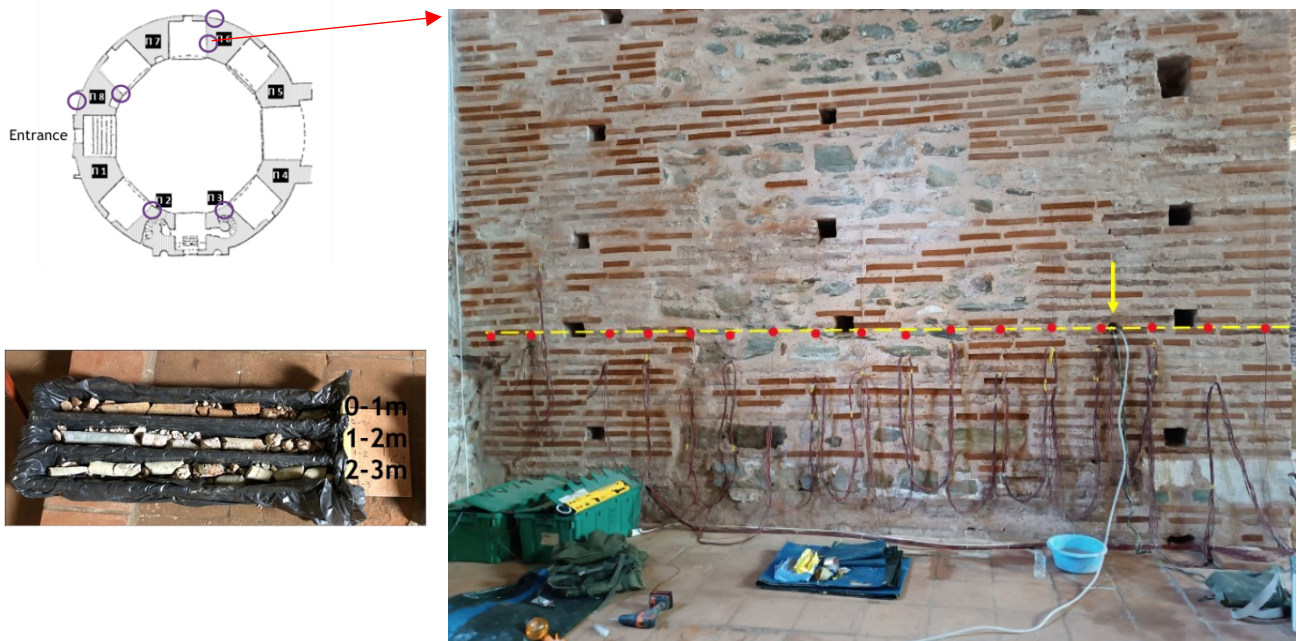
Figure 5.3: Photograph of the investigated wall (on the right). The dashed yellow line indicates the reference plane where the surface electrodes (red dots) are situated. The arrow points to the tip of the borehole. On the top left corner there is the top view of the monument and on the bottom corner a picture of the borehole's core.
