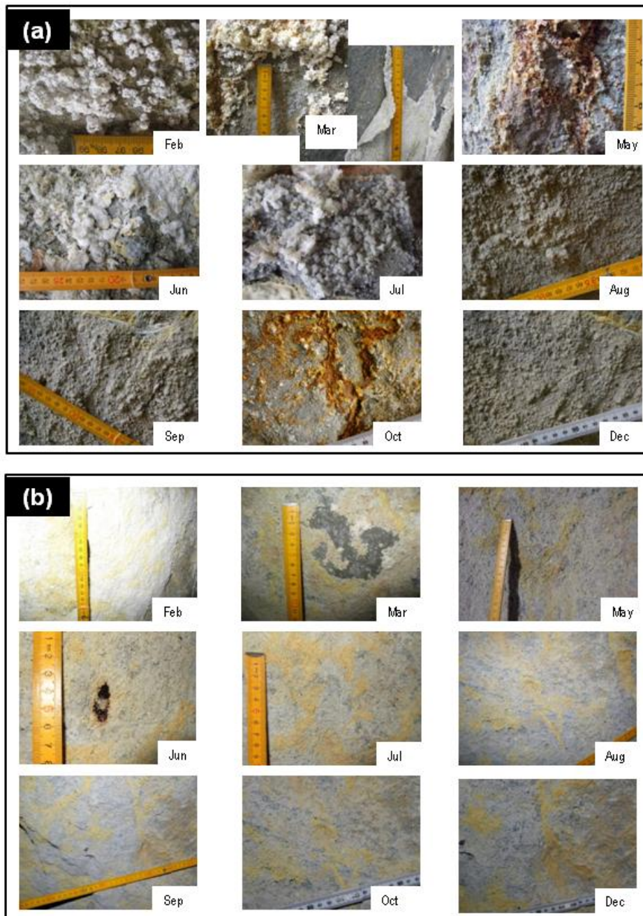
Fig. 4. Salt efflorescence of the rock wall. (a) Point 2 and (b) Point 8.
